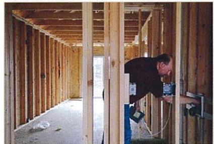
Rick Bramall, chief plans examiner for Springdale, inspects a new home Thursday on Rosemary Avenue in Springdale. The builder could request inspections online, if the city's Building Department switches software. Photo by Sarah Bentham
